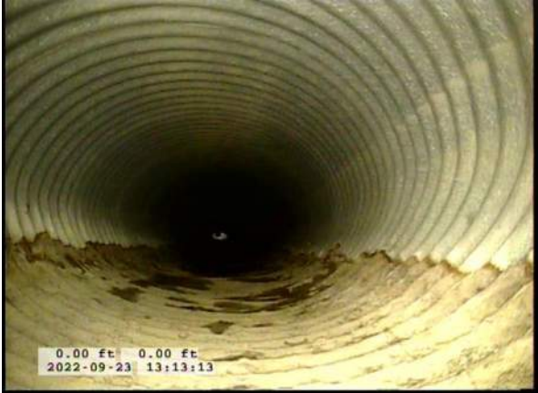
1, 00:00:09, 0.00ft Catch Basin / CB3
