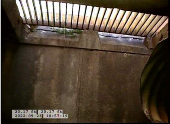
9, 00:02:33, 20.17ft Catch Basin / CB8
