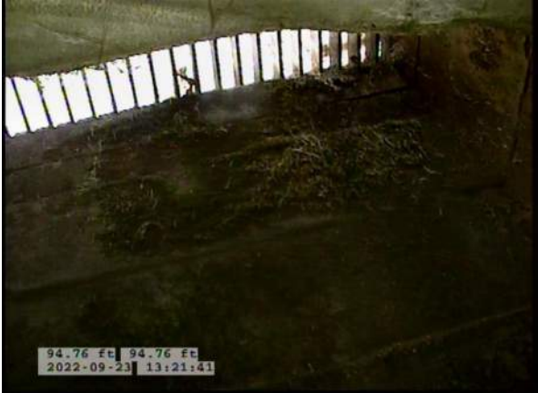
9, 00:07:26, 94.76ft Catch Basin / CB2
