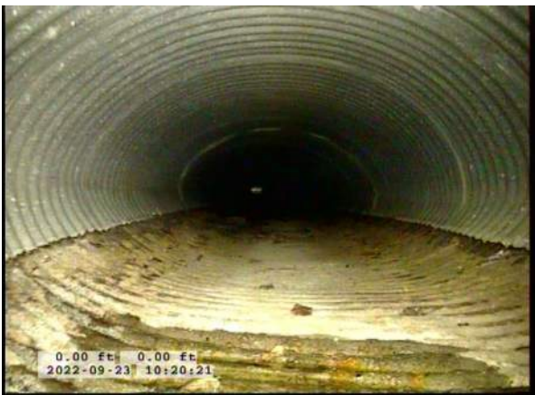
3, 00:00:18, 0.00ft Deposits Attached Encrustation, 5% of cross sectional area from 5 o'clock to 7 o'clock, within 8 inch, Start / RUST
