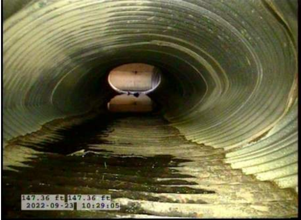
13, 00:07:00, 147.36ft Deposits Settled Compacted, 5% of cross sectional area from 5 o'clock to 7 o'clock, within 8 inch, Finish
