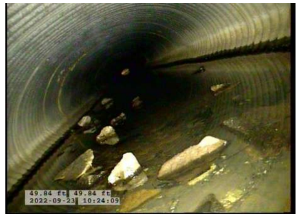
8, 00:03:22, 49.84ft Deposits Settled Compacted, 5% of cross sectional area from 5 o'clock to 7 o'clock, within 8 inch, Finish
