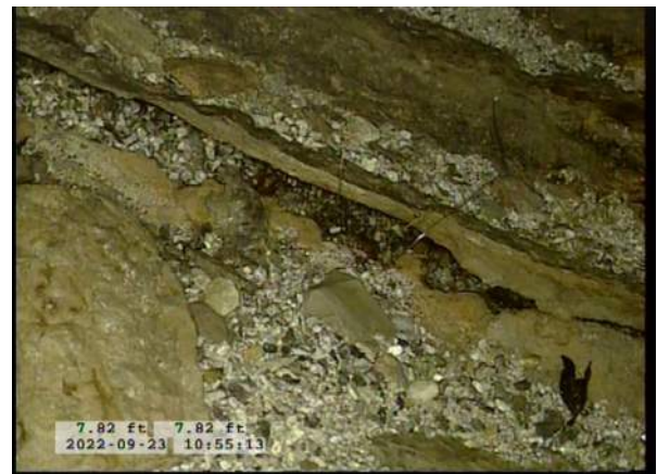
4, 00:01:06, 7.82ft Surface Damage Missing Wall from 5 o'clock to 7 o'clock / BOTTOM OF PIPE STARTING TO RUST AWAY
