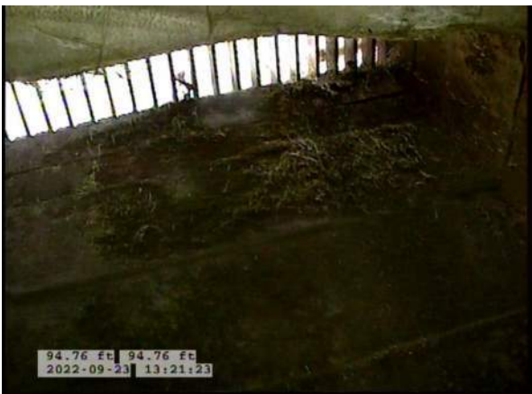
7, 00:07:20, 94.76ft Deposits Attached Encrustation, 5% of cross sectional area from 5 o'clock to 7 o'clock, within 8 inch, Finish / RUST
