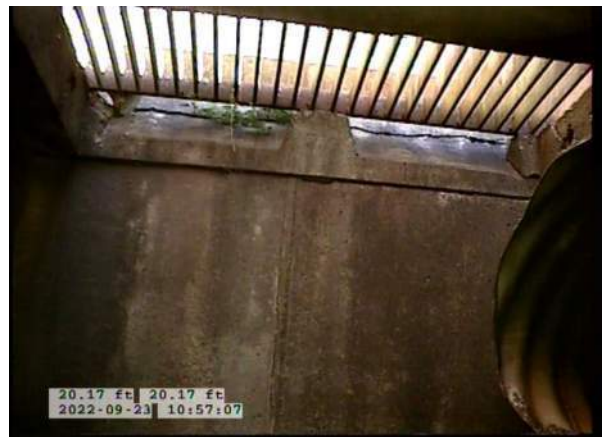
8, 00:02:30, 20.17ft Deposits Attached Encrustation, 5% of cross sectional area from 5 o'clock to 7 o'clock, within 8 inch, Finish
