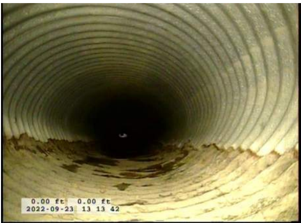
3, 00:00:17, 0.00ft Deposits Attached Encrustation, 5% of cross sectional area from 5 o'clock to 7 o'clock, within 8 inch, Start / RUST
