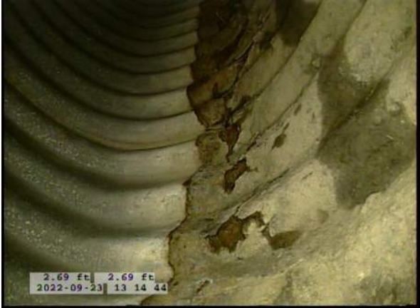
5, 00:00:44, 2.69ft Surface Damage Missing Wall from 5 o'clock to 7 o'clock, within 8 inch, Start / BOTTOM OF PIPE HAS BEGUN RUSTING AWAY
