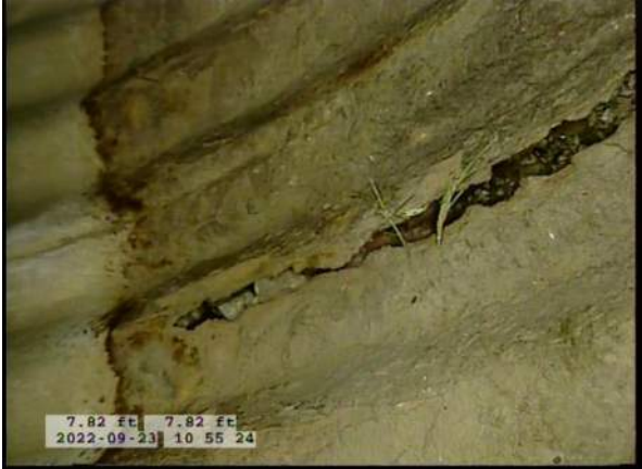
5, 00:01:06, 7.82ft Surface Damage Missing Wall from 5 o'clock to 7 o'clock / BOTTOM OF PIPE STARTING TO RUST AWAY
