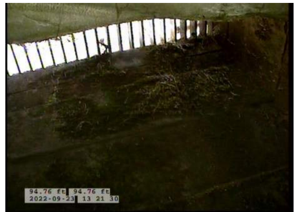
8, 00:07:23, 94.76ft Surface Damage Missing Wall from 5 o'clock to 7 o'clock, within 8 inch, Finish / BOTTOM OF PIPE HAS BEGUN RUSTING AWAY
