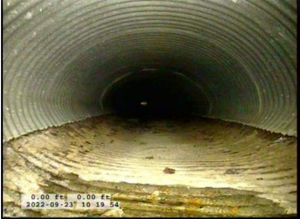
1, 00:00:11, 0.00ft Catch Basin / CB9
