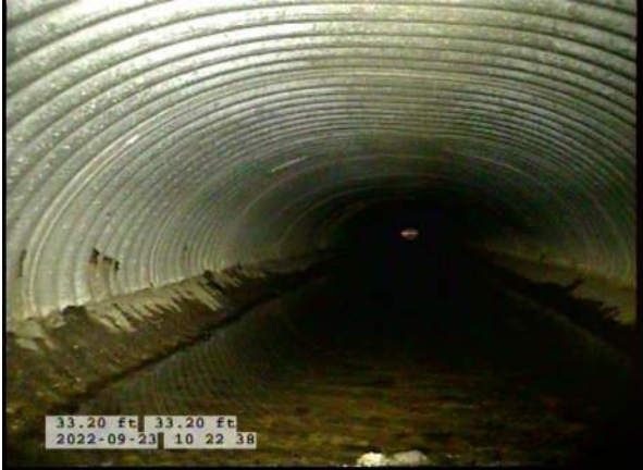
5, 00:02:12, 33.20ft Deposits Settled Gravel, 5% of cross sectional area from 6 o'clock to 7 o'clock, within 8 inch, Finish
