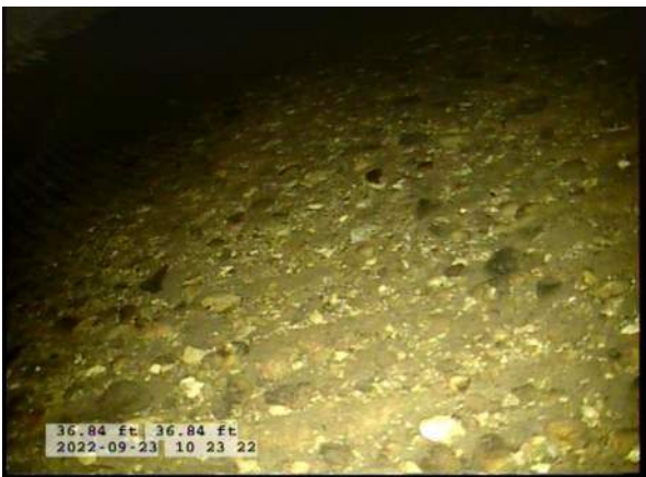
7, 00:02:37, 36.84ft Deposits Settled Compacted, 5% of cross sectional area from 5 o'clock to 7 o'clock, within 8 inch, Start
