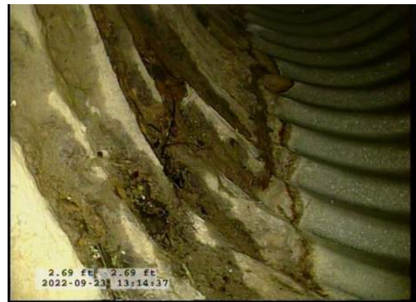
4, 00:00:44, 2.69ft Surface Damage Missing Wall from 5 o'clock to 7 o'clock, within 8 inch, Start / BOTTOM OF PIPE HAS BEGUN RUSTING AWAY
