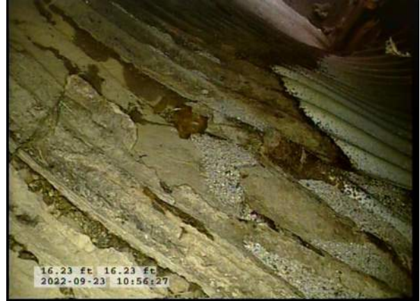
6, 00:01:53, 16.23ft Surface Damage Missing Wall from 5 o'clock to 7 o'clock / BOTTOM OF PIPE RUSTING AWAY
